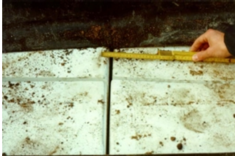
Figure 3. Relative horizontal movement and a resulting gap of approximately 20 mm between blocks of EPS geofoam used as lightweight fill in the Matlingeweg street reconstruction project in Rotterdam, The Netherlands. This movement occurred within an portion of the street with a single layer of geofoam blocks and contributed to premature failure of the overlying asphaltic concrete pavement after one month of service (courtesy of Dr.-Ir. Milan Duškov of Oranjewoud International).
