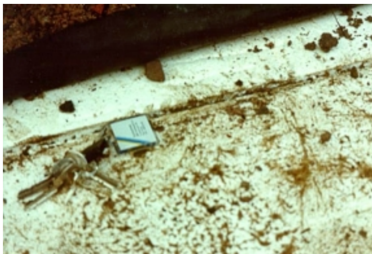
Figure 2. Relative vertical movement of approximately 5 mm between blocks of EPS geofoam used as lightweight fill in the Matlingeweg street reconstruction project in Rotterdam, The Netherlands. This movement occurred within an portion of the street with a single layer of geofoam blocks and contributed to premature failure of the overlying asphaltic concrete pavement after one month of service (courtesy of Dr.-Ir. Milan Duškov of Oranjewoud International).
