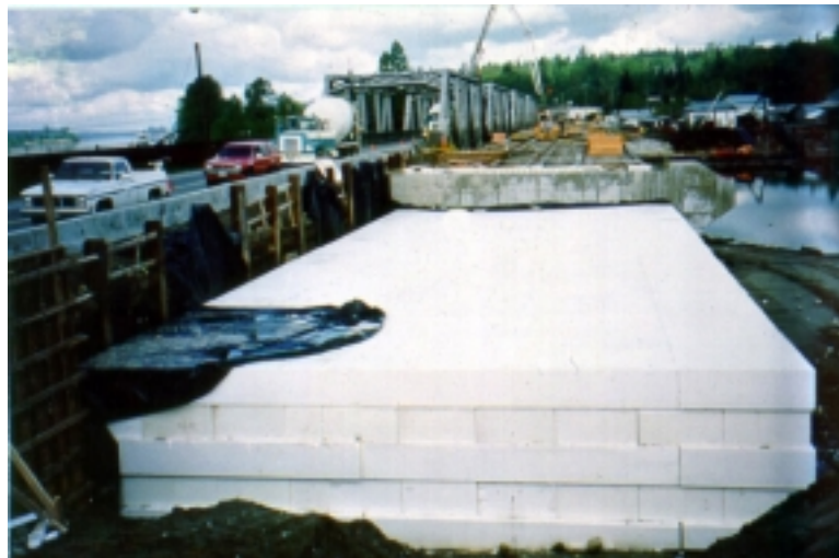
Figure 4. New bridge approach fill under construction utilizing EPS-block geofoam as lightweight fill on Highway 7 at the Stave River in British Columbia, Canada. Important design details such as multiple layers of geofoam blocks and alternating block orientation, both of which contribute to the individual geofoam blocks acting as a single homogeneous mass, are illustrated (courtesy of Mr. Michael Tobin of AFM ® Corporation).
