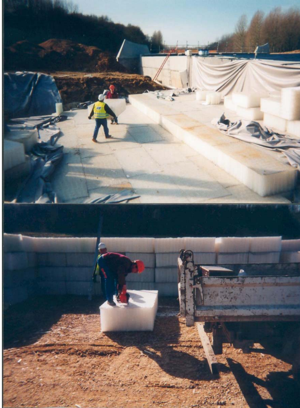
FIG. 4. Geocomb Blocks Used as Lightweight Fill on a Bridge Project in France
