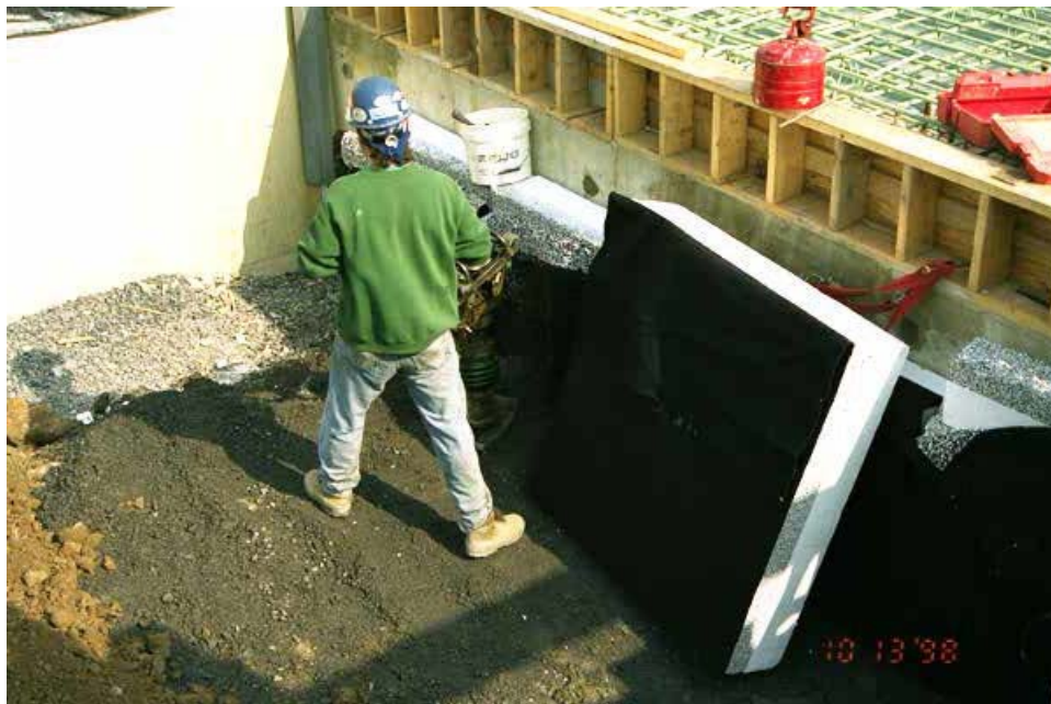
FIG. 2. Geofom Geocomposite Used as a Compressible Inclusion on a Bridge Project in the Commonwealth of Virginia, U.S.A.
