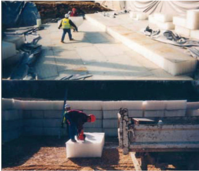
Figure 5. PP-Geocomb Blocks Used as Lightweight Fill on a Bridge Project in France.
